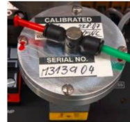
Figure 6 Pressure Test Point
